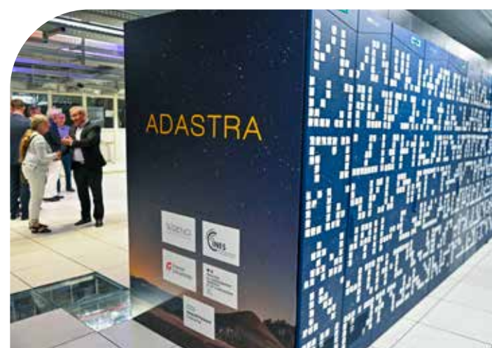
At the CINES facility in Montpellier.
